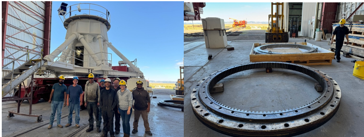
(Left) Subset of the Engineering Services team performing the azimuth bearing replacement on Antenna 12; (Right) old (bottom) and new (top) bearings for Antenna 12.
