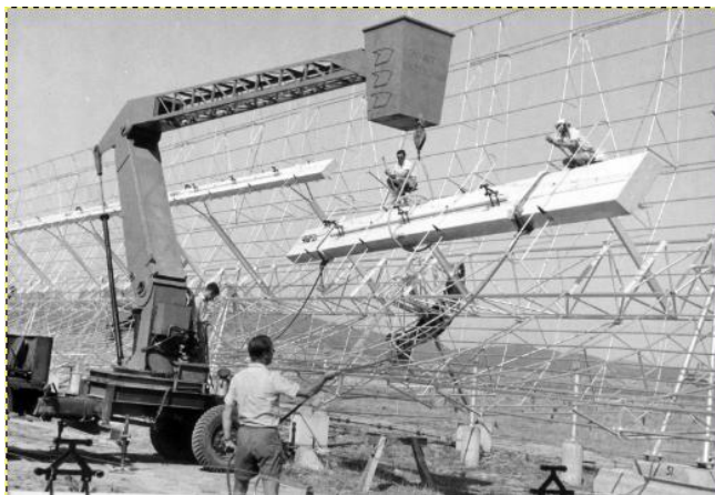
Lifting the feed on the east-west arm into position during the building of the Molonglo Cross in 1965.
