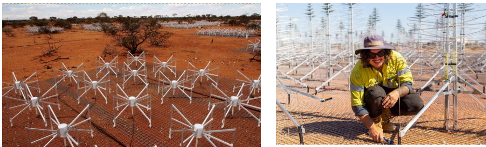
Left: the Murchison Widefield Array (MWA); right: installing antennas of the Aperture Array Verification System, a testbed for SKA-Low, at the MWA site. Credits: ICRAR/Curtin University
