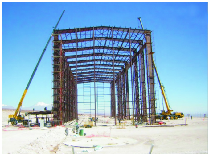
Figure 4. The VertexRSI antenna site erection facility building rises on the OSF grounds. Antennas will be assembled in this large facility which is nearly eight stories tall.
