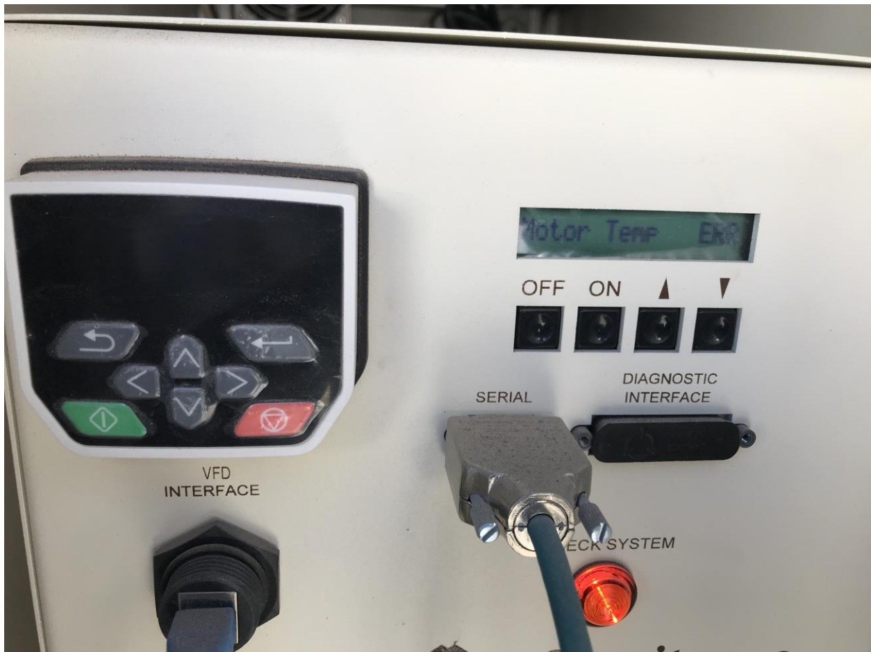
Picture 38: Motor Temp Err is displayed after the compressor's shutdown
