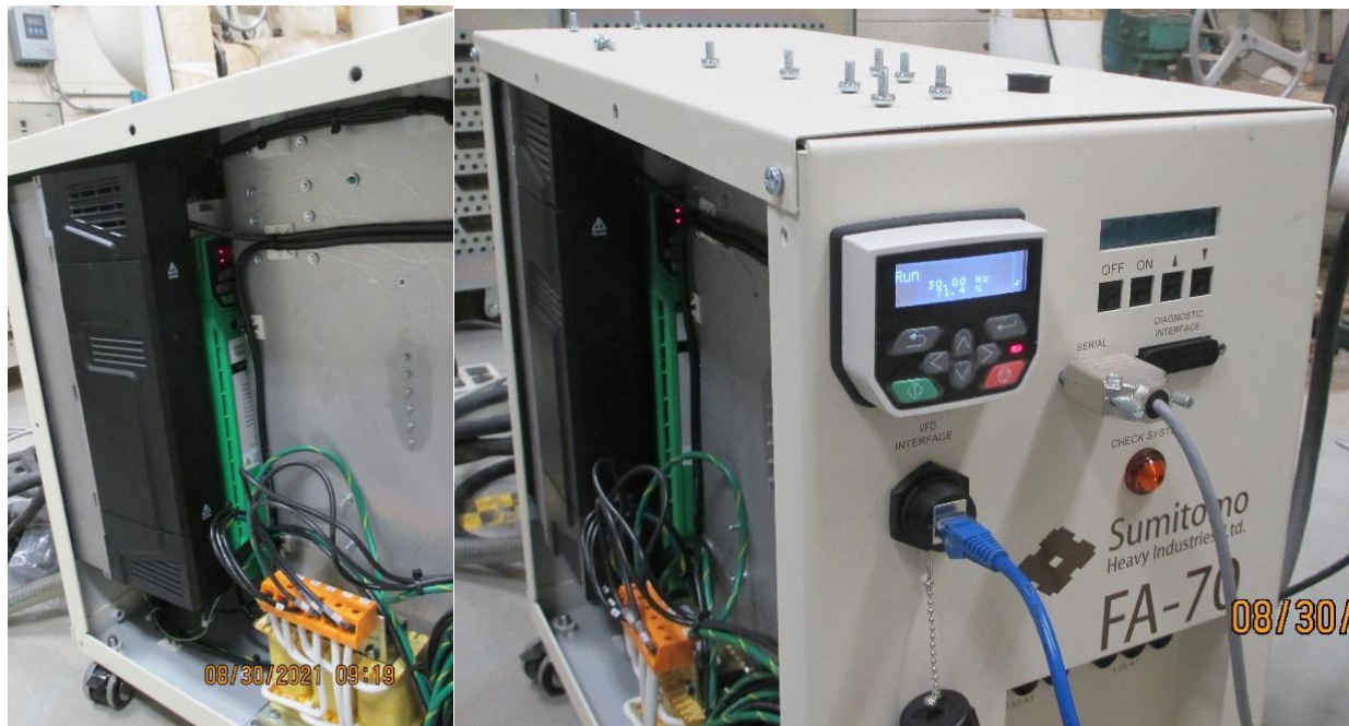
Picture 22: Integration of the Inverter with Indoor Compressor Unit (ICU)
