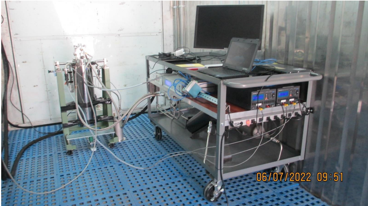
Picture 31: Cryo-Test Cart and Sumitomo Test Cryostat Installation Inside the Container
