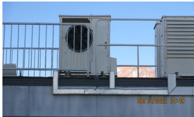
Picture 34: Enclosure with louver removed showing the compressor fan.
