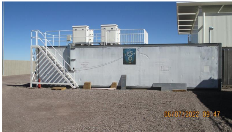
Picture 30: Container with Compressor Enclosures Mounted on the Roof at the OSF
