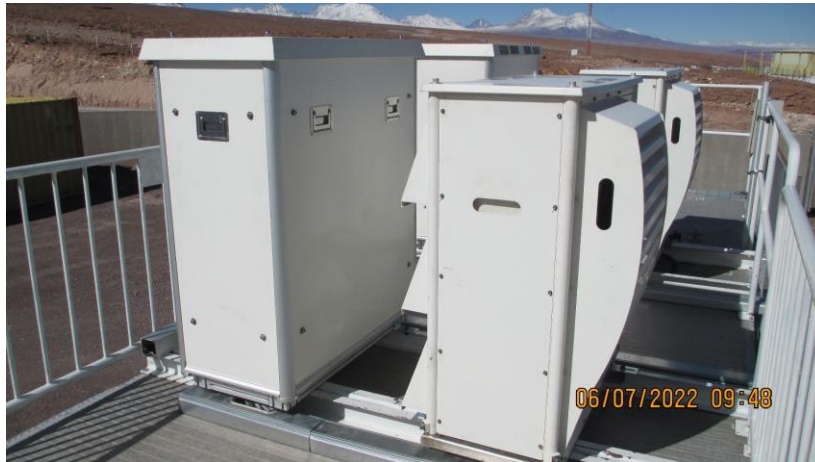
Picture 29: Enclosure for the ICU on the Left and OCU Enclosure on the Right
