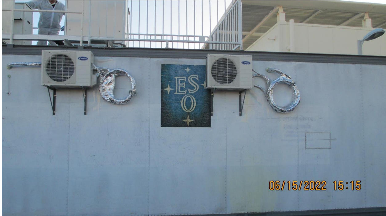
Picture 33: Two Heat Pumps Mounted on the Side of the Container to Control the Inside Temperature
