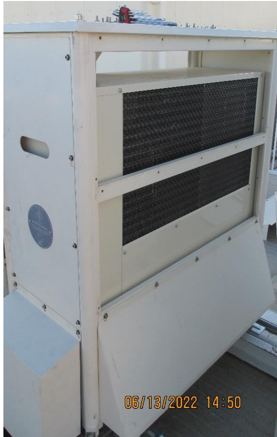
Picture 35: Sides of the Outdoor Enclosure Removed to Test Impact on the Power Consumption
