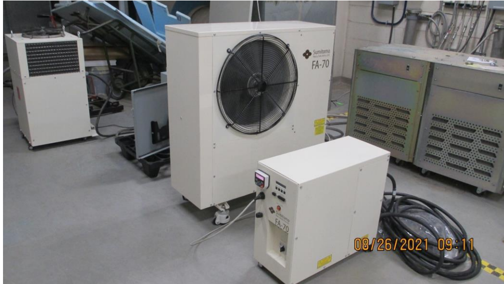
Picture 27: Sumitomo FA-70V Compressor Installed in DSOC Mechanical Room
