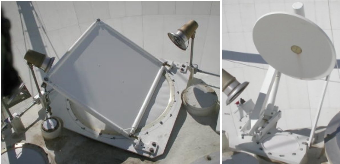
The dichroic panel is in good condition. The dish tipper overtravel springs were replaced because they were showing some rust.
