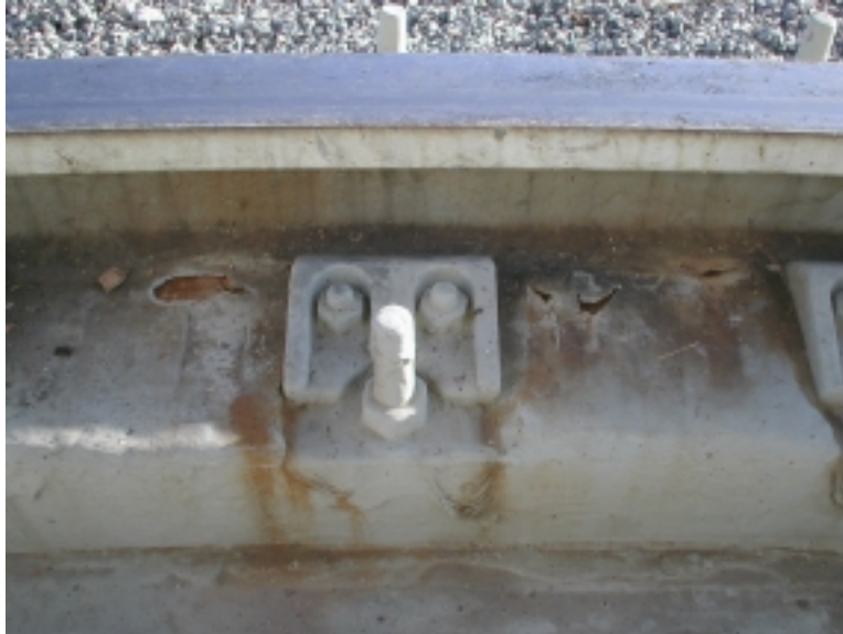
The azimuth rail grout and Vulkem are in good condition, but the grout is crumbling in a few areas.
