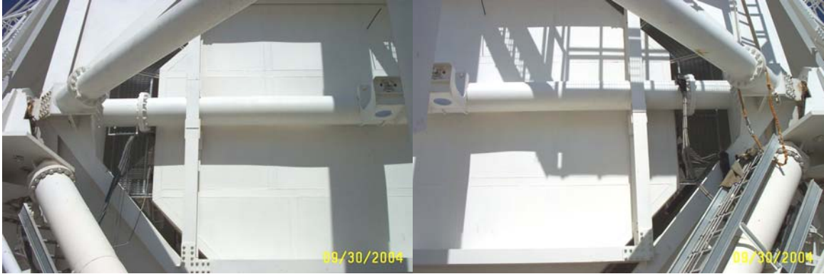
Elevation axle has no visible signs of cracks. Paint is in excellent condition.
