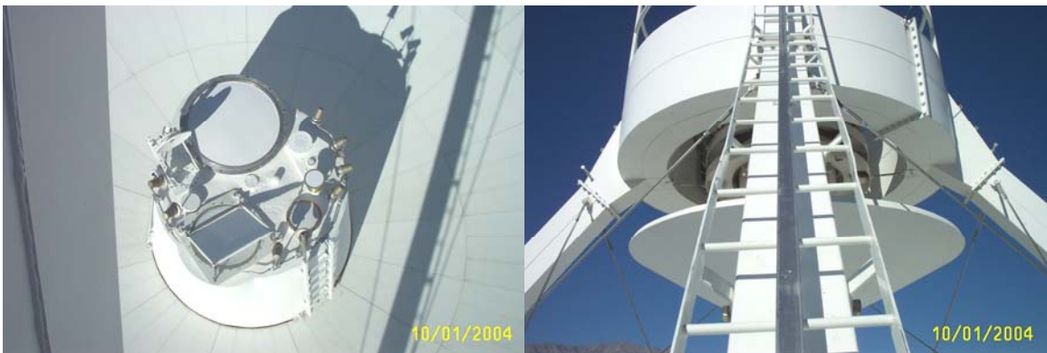
Feed cone and feed windows are in good condition. Apex paint is excellent.
