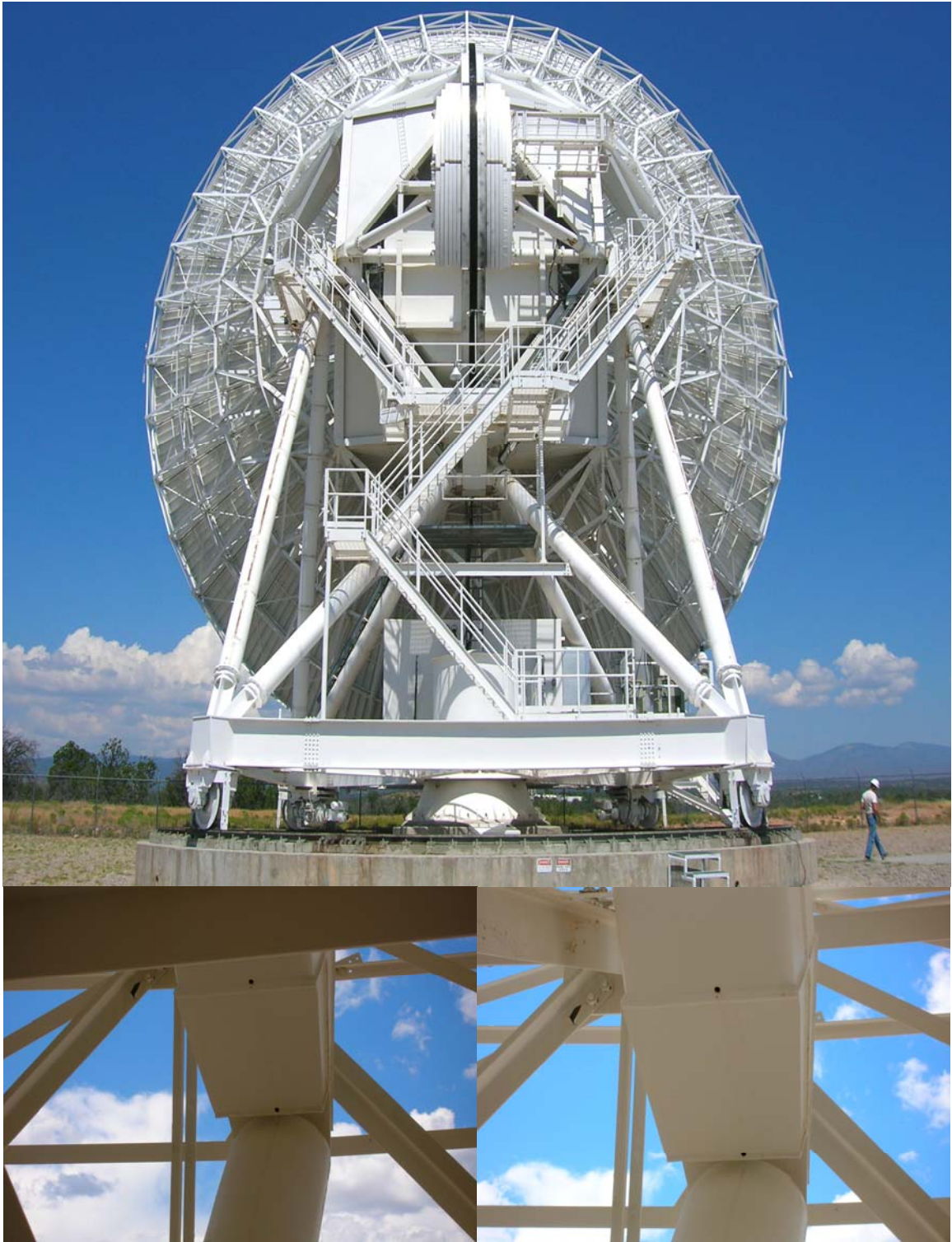
Overall the paint on the Los Alamos antenna is in good condition. Notice the drain holes drilled in the Quad Legs.
