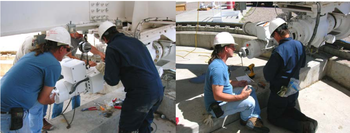
Elevation #2 and azimuth #1 motors were replaced. Digital tachometers were installed and calibrated on the azimuth and elevation motors.
