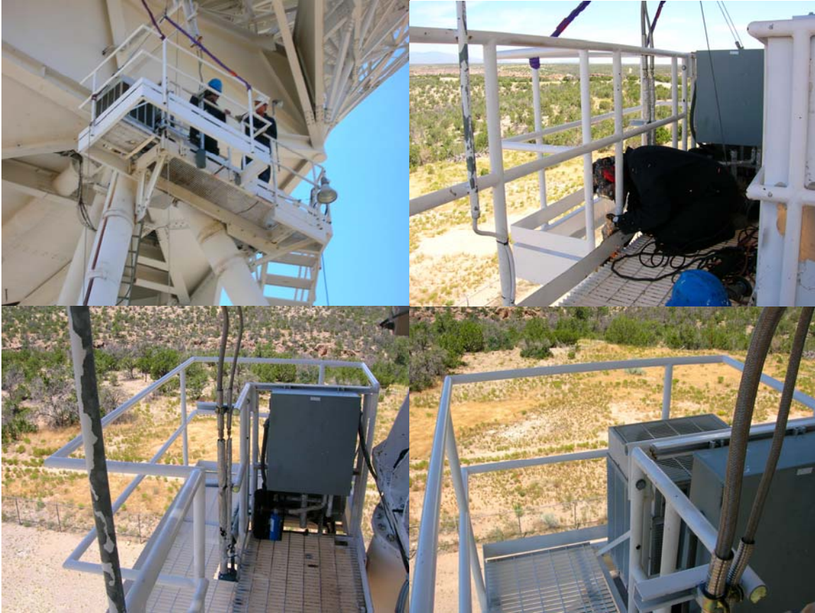
A new HVAC platform extension was installed. Maintenance performed on the vertex room compressor/condenser can now be completed safely.
