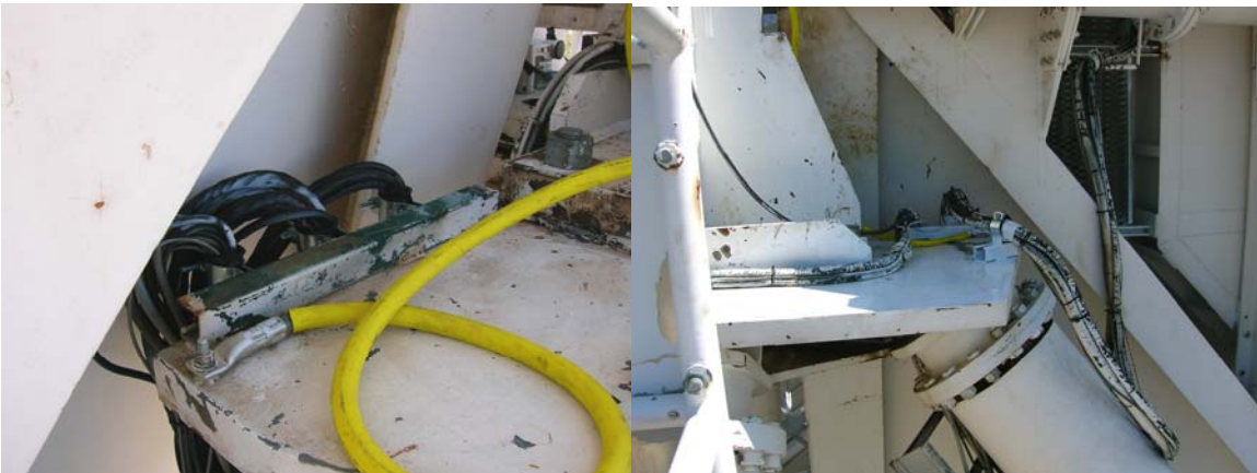
Both the encoder and synchro side elevation cable wraps were repaired by repositioning and replacing strain relief brackets. Both sides elevation ground cables were replaced.
