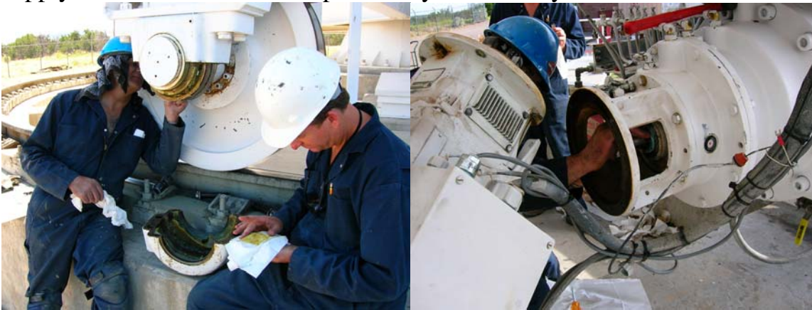
Azimuth wheel bearings were inspected. Azimuth #2 gear box seal was replaced with a double seal setup.
