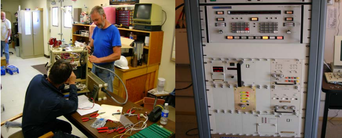
The ACU backplane upgrade was installed and tested. The ACU power supply modification had been previously installed by Paul Johnson.
