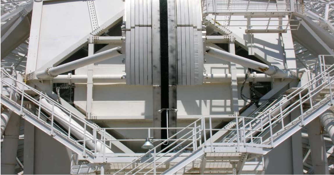
Elevation axle has no visible signs of cracks. Paint is in good condition.
