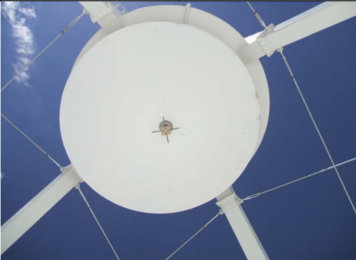
Sub reflector is in excellent condition
