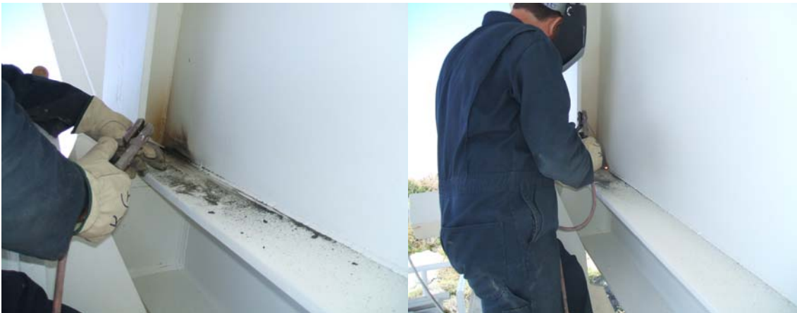
A four inch crack was repaired above the synchro side elevation axle.
