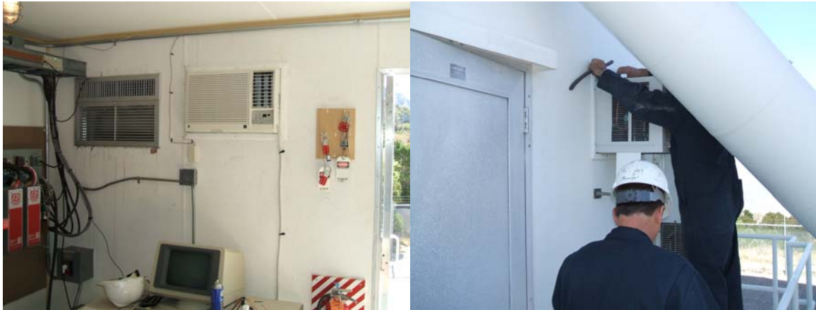
A new back up AC was installed for the Pedestal room electronics.
