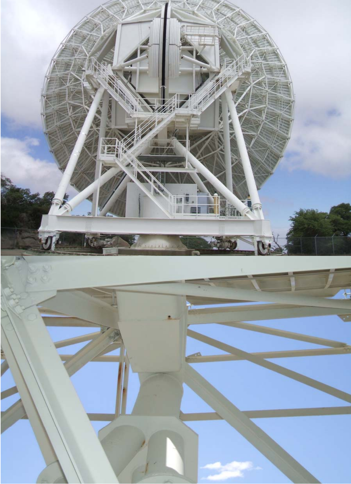
Overall paint on the antenna is in excellent condition with only a few surface rust spots. Notice the Quad leg drain hole.
