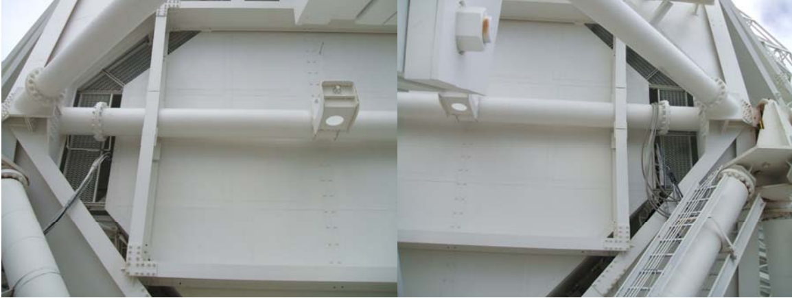
Elevation axle has no visible signs of cracks. Paint is in Good condition.
