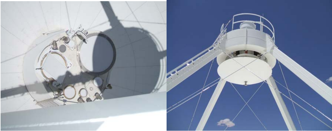
Feed heaters and FE windows are in good condition. Apex paint is in good condition.
