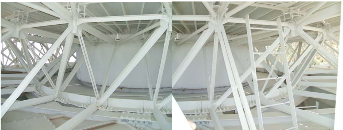
Antenna backup structure is in good condition. Paint is in good condition
