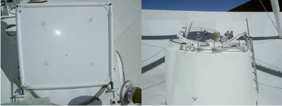
Dichroic reflector is in good condition. Ellipsoid reflector is in good condition and operates correctly.
