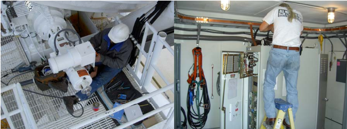
The New Digital Tach modification was completed and the Site Techs were trained on tach calibration for both axis. The Azimuth stair step emergency stop cable was replaced. The Snake Pit door interlock was also repaired.
