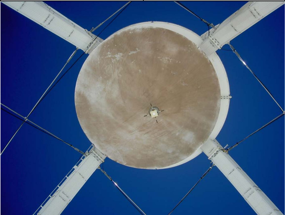
Sub reflector paint is discolored.
