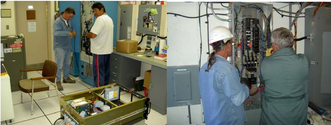
The MKV recorder and its communications were put on UPS power with the addition of a new terminal block mounted underneath the floor in room 103. Both MKIII recorders were removed. Inside the Servo drive cabinet and the Ped Room power panels many loose connections were found.
