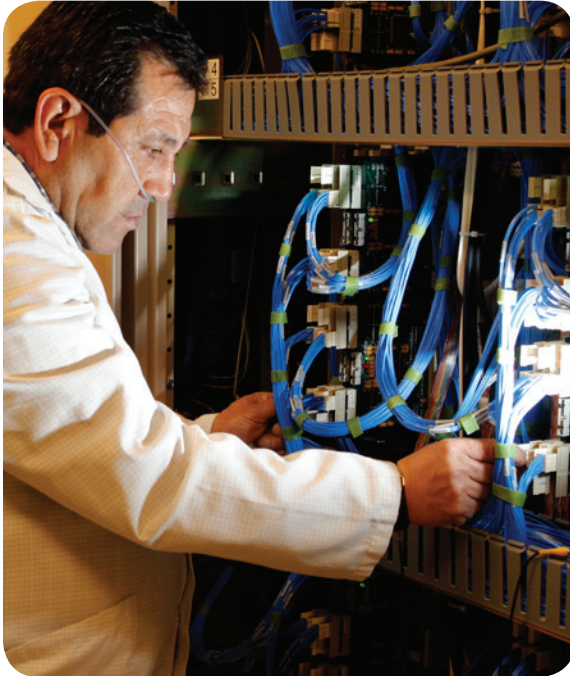
Technician Juan Carlos Gatica checks electronics on the ALMA correlator while using supplemental oxygen at the high-altitude site (Carlos Padilla, NRAO/AUI/NSF).
